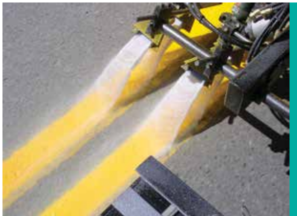
Figure 16. Glass beads being applied during a double-yellow-centerline plural-component epoxy application (Image: ATSSA Pavement Marking Division)
