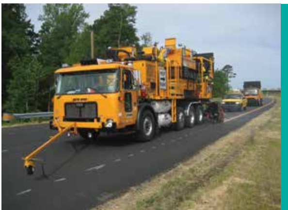
Figure 15. Yellow spray thermoplastic edge lines being applied to an interstate highway near Raleigh, N.C. (Image: ATSSA Pavement Marking Division)
