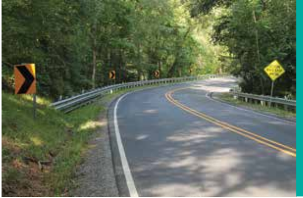
Figure 6. Post-mounted chevrons in a curve, Route 218, King George County, Va. The school-area sign (right) warns of pedestrians in the area (Image: James Scott Baron, ATSSA)
