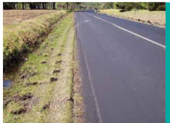
Figure 20. Note the tire tracks on the shoulder and onto the roadway. The edge of the Safety Edge SM remained unharmed after being crossed by a fully loaded asphalt truck during road construction (Image: Frank Julian, FHWA)
