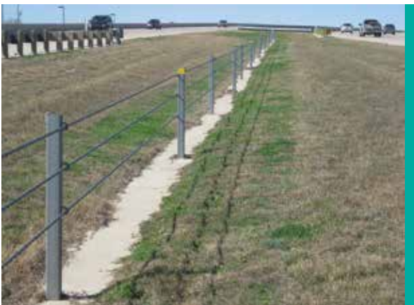
Figure 31. Installed cable median barrier (Image: Gibraltar)
