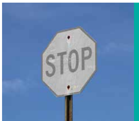
Figure 4. Faded, ineffective signs like this should be replaced to immediately improve roadway safety for motorists (Image: James Scott Baron, ATSSA)
