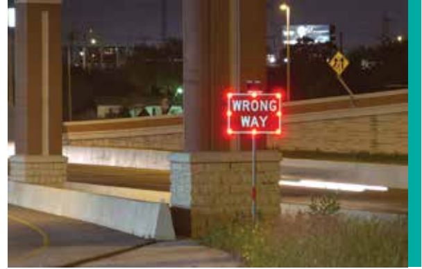
Figure 7. A Wrong Way sign with LED enhancement (Image: Traffic & Parking Control Co. Inc. (TAPCO))
